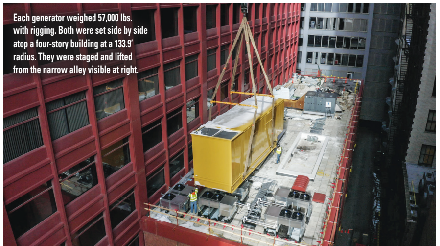
Each generator stood 40'4" long, 10'8" wide, and 13'2" high. The crane operator had only 3'6" of clearance on each side as he hoisted a generator.
